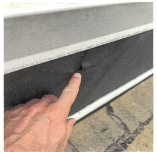
Tall vertical walls have EPDM waterproofing and need repairs
