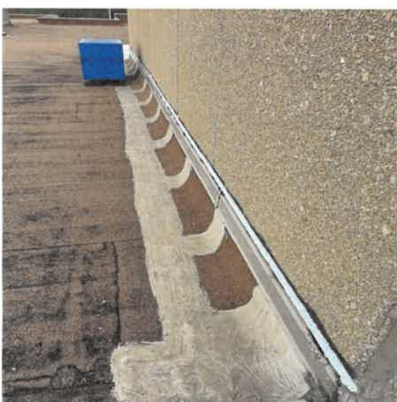
Wall flashings and metal trim are in poor condition and need to be replaced.
