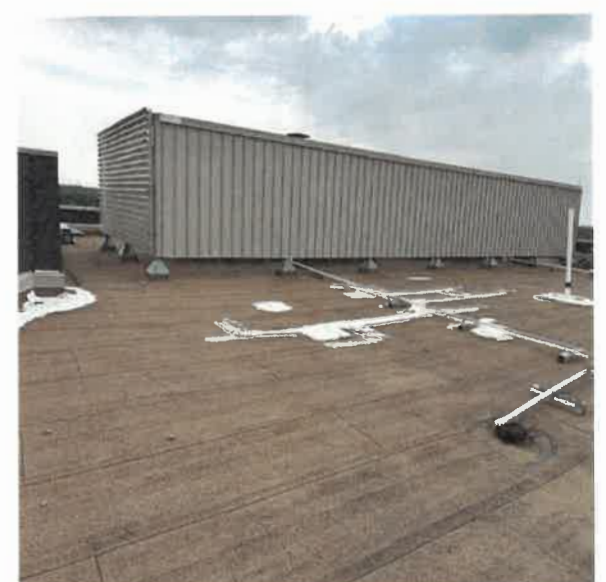
Additional patch area indicating leak in field and/or flashings
