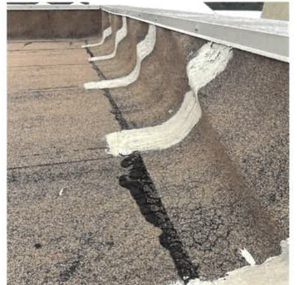
Recommend replacement of wall flashings and coping cap metal.
