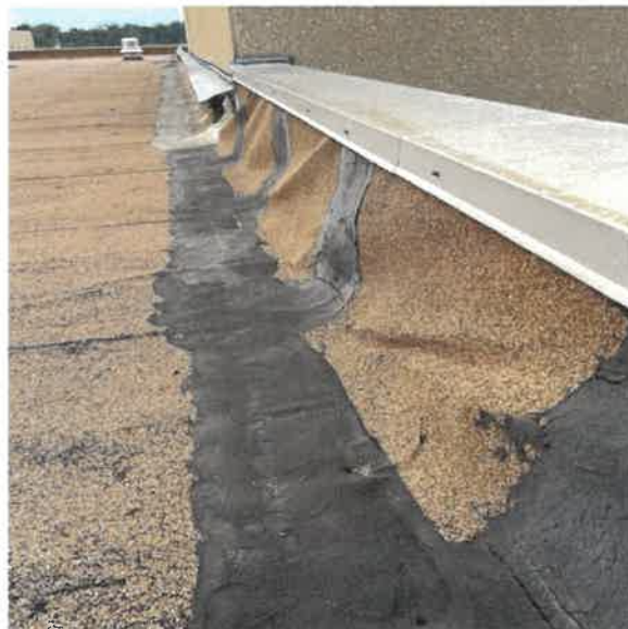
Detached wall flashings were found throughout roof system.
