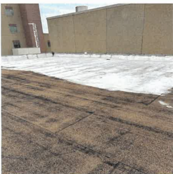
Noted areas of patching indicating leak and potential wet insulation
