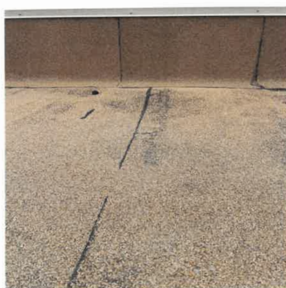
Noted blisters that would require patching prior to restoration.
